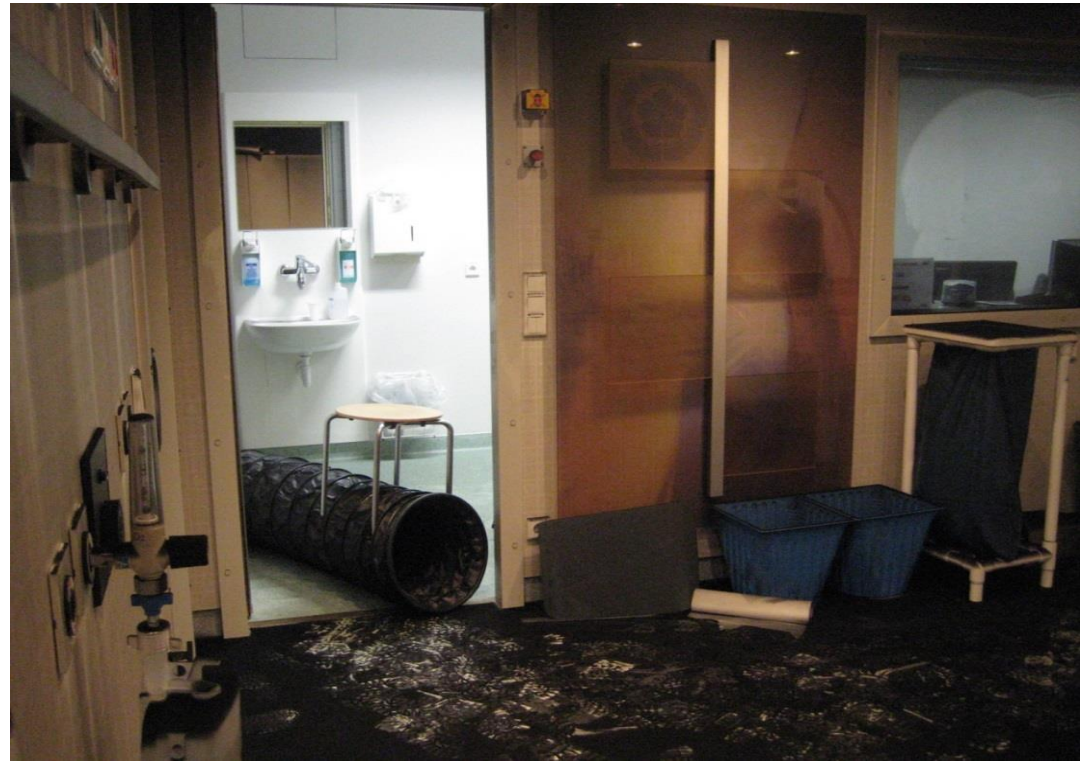
26.10.2009 – Würzburg Fire in Hospital
